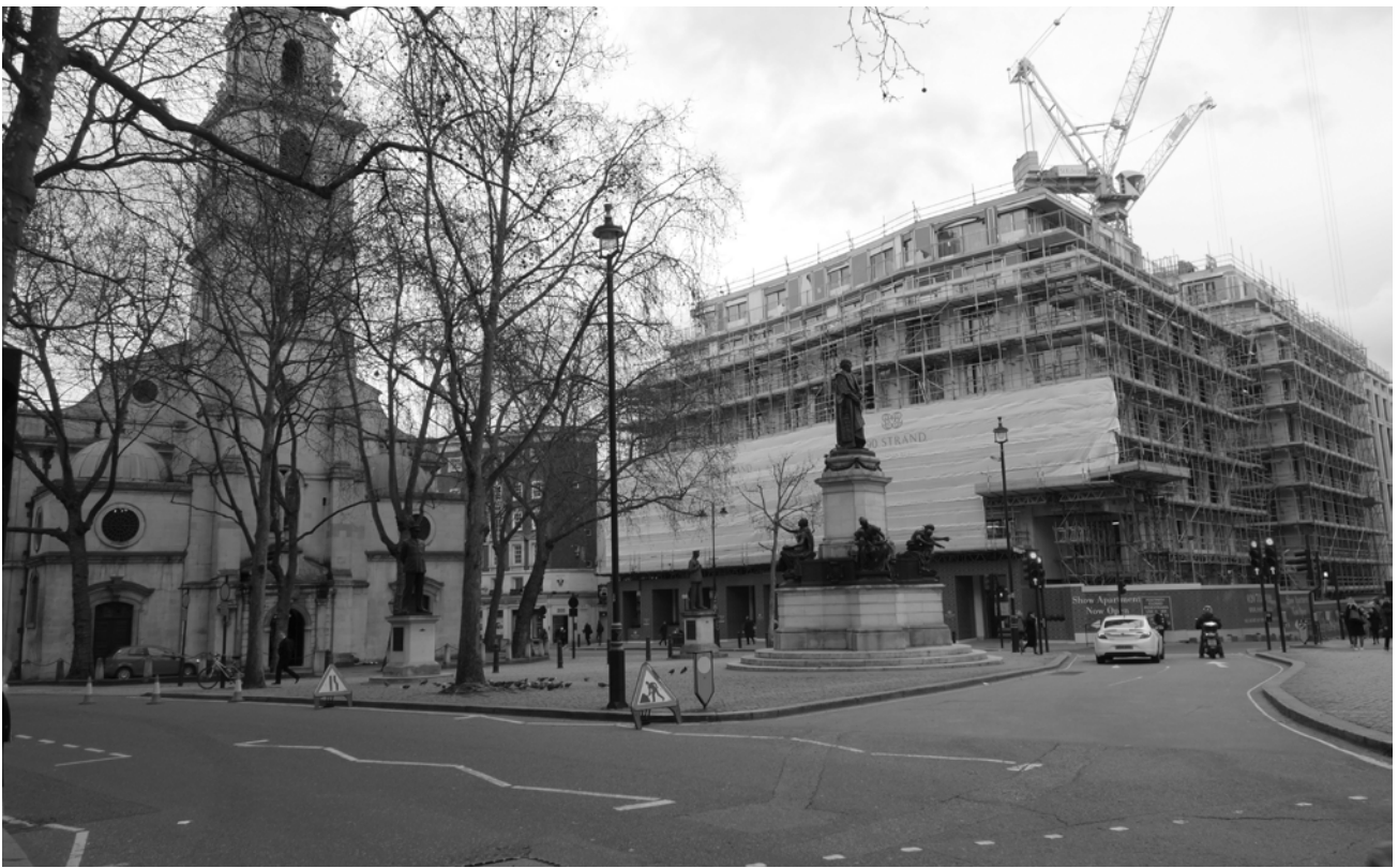
View south east from the Aldwych towards St Clement Danes and 190 Strand
