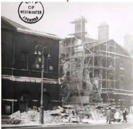
Fig.24 Damage to Paymaster General's Office, Whitehall, 8th October 1940. (Content edited by Community Sites (www.communitysites.co.uk), no date c)
