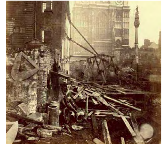
Fig.13 Site clearance prior to excavation work for Westminster Station c.1866. (Flather H. C1866).
